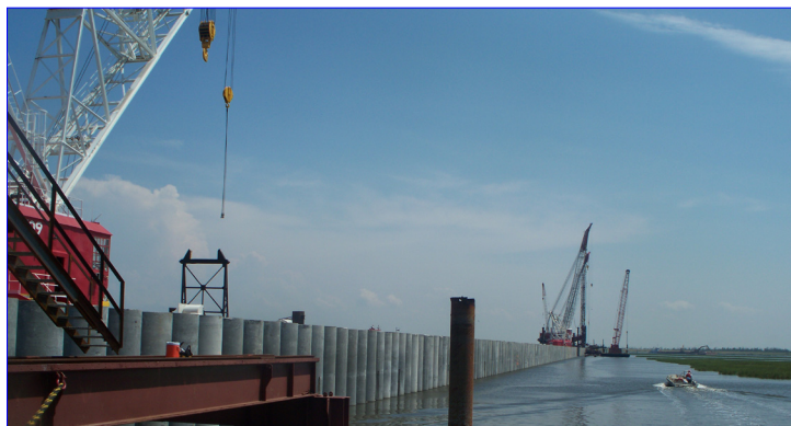
Concrete Cylinder Piles form the New Orleans IHNC Floodwall; Work Trestle in foreground. Photo courtesy of Foundation Testing and Consulting.
