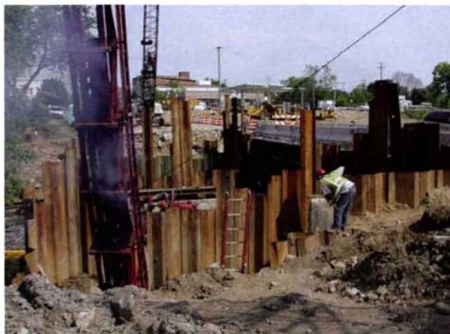
Work proceeds on the Main Street Bridge project in Scio Township near the village of Dexter.
