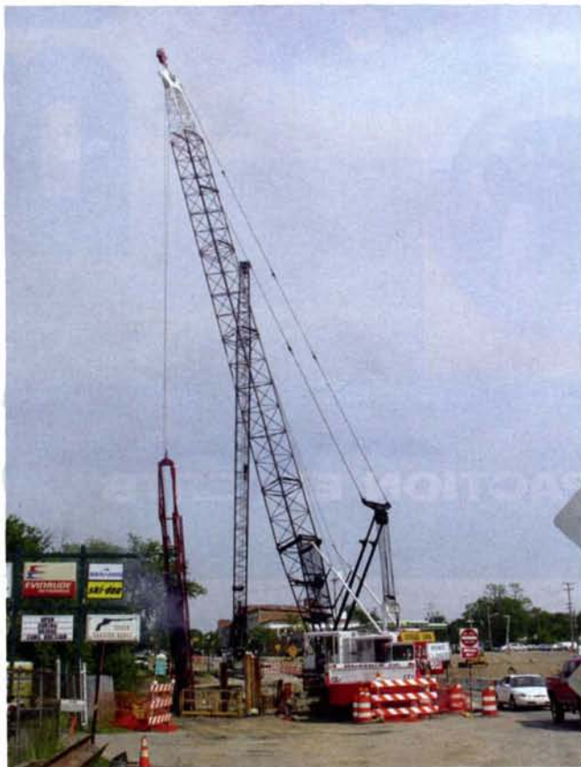
MacKenzie's 85-ton Link-Belt crane drives H-pile for the Main Street Bridge replacement project in Scio Township near the village of Dexter.
