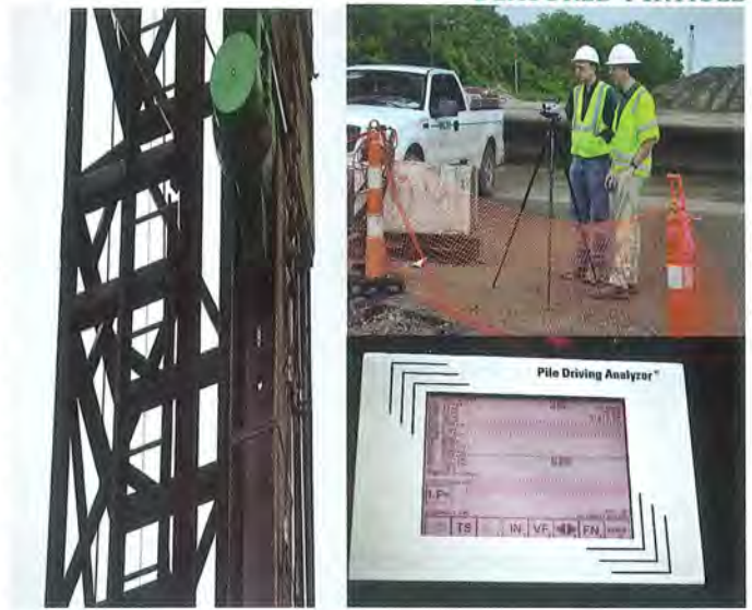
Figure 3: PDA instrumentation on an HP 18x204 and GRL Engineers' Dr. Brent Robinson (left) and Eric Bogen video recording while the PDA Model PAX processes the pile data.
