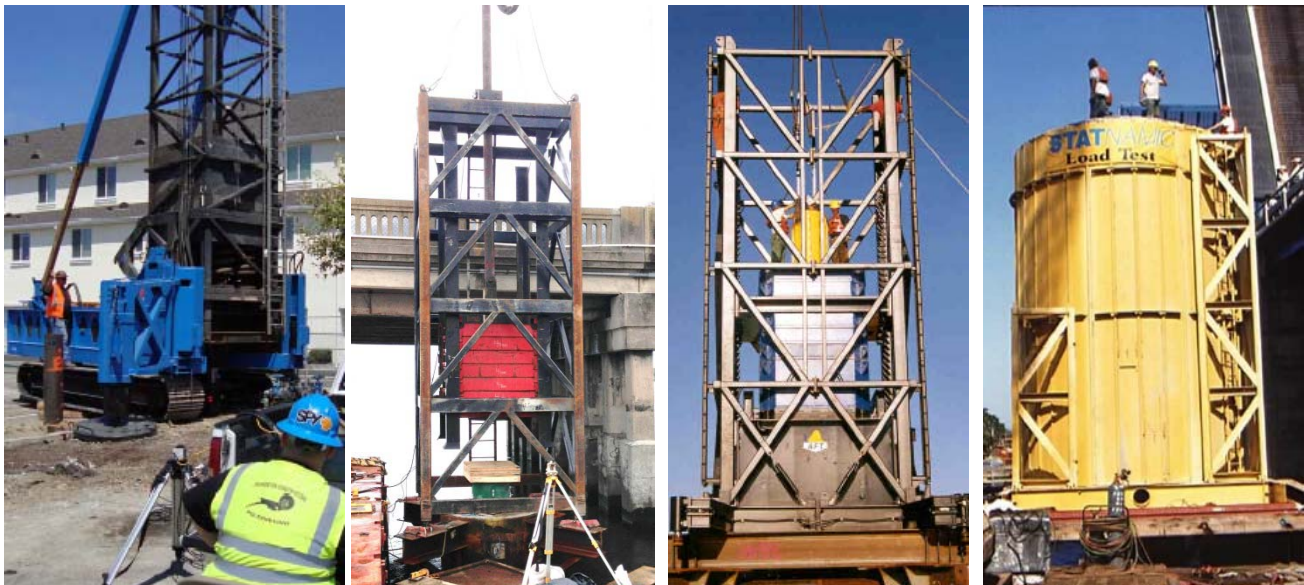
Figure 16: (a) Fundex mass with heavy spring cushion, (b) cushioned dynamic test, (c) Statnamic with catch mechanism, (d) Statnamic with gravel containment housing (for larger loadings)
