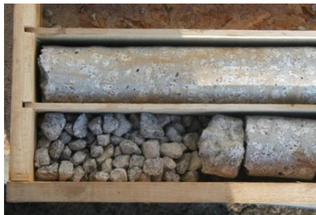
Figure 4: core of the defective shaft
