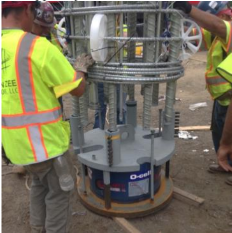
Figure 13: hydraulic jack attached to bottom of reinforcing cage of a bored pile
