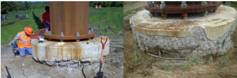
Figure 1. Fill placed around and pushed under top form created a void at ground level
