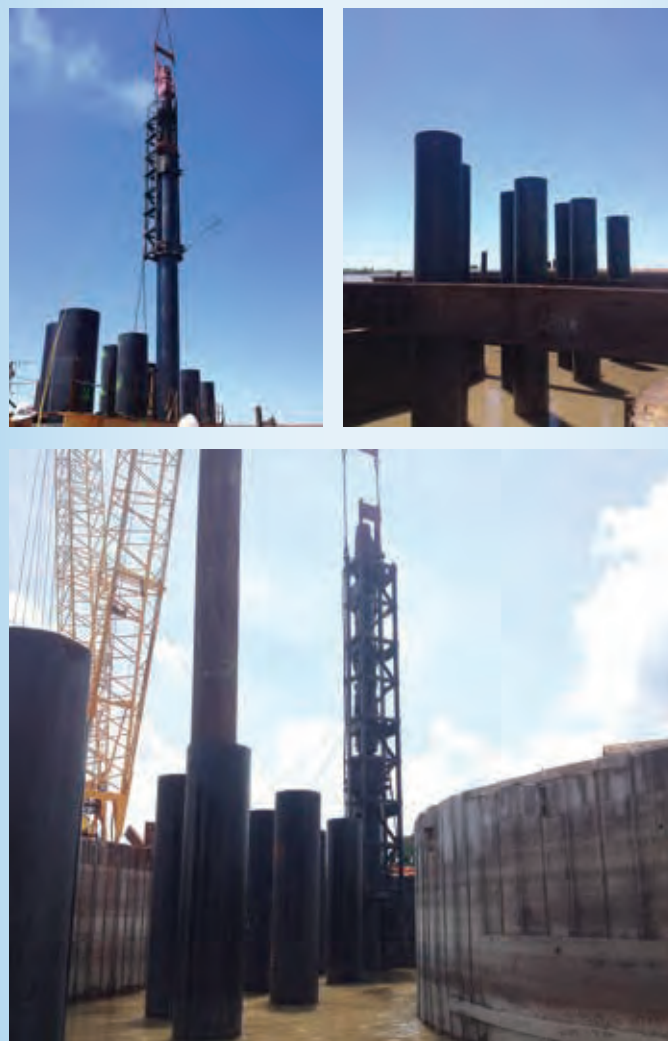
Figure 2 – PILECO D100 installing pipe piles to tip elevation on the Mississippi River
