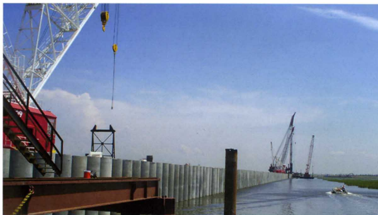
Concrete Cylinder Piles form the New Orleans IHNC Floodwall; Work Trestle in foreground.
