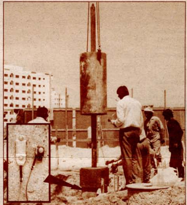
PDA test of Drilled Shaft (Photo courtesy of Dr. M. Mukaddam, I&M, Dubai, UAE)
