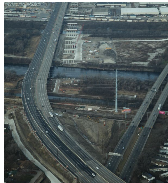
Figure 1: Aerial View of Mile Long Bridge During Construction – Photo Courtesy of Brian Fritz Photography
