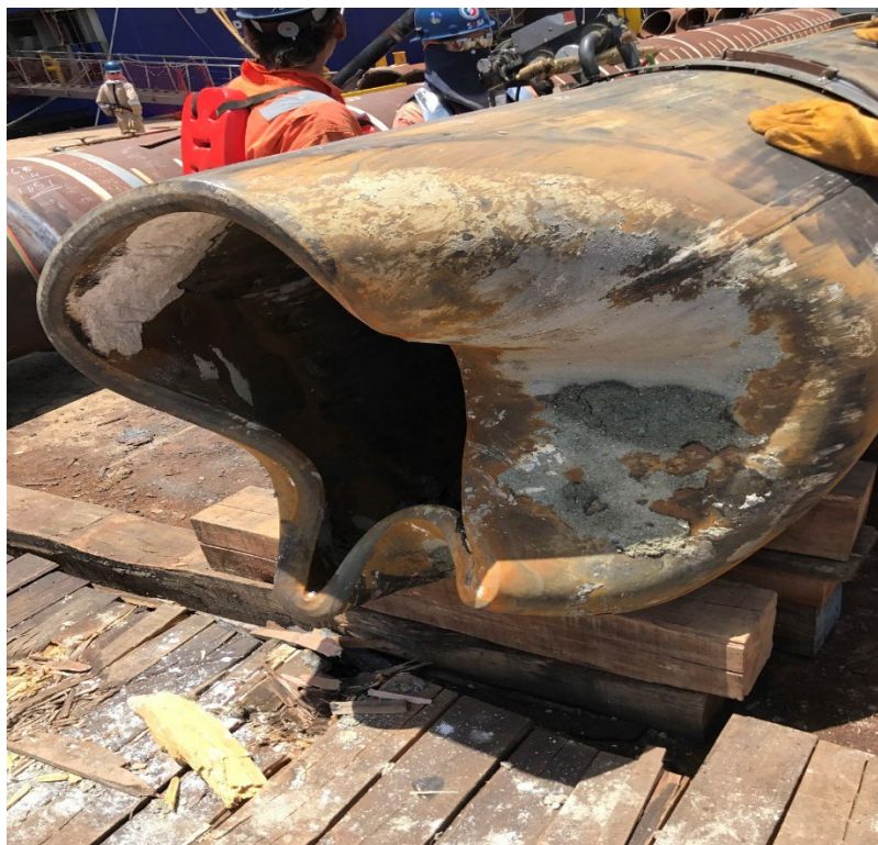
Figure 2 – Pile toe damage
