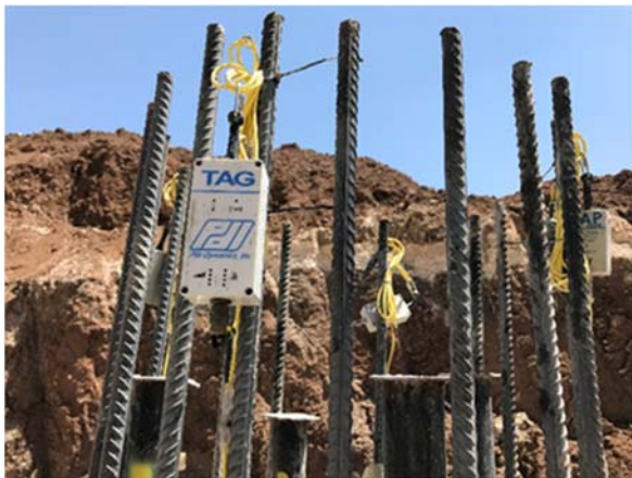
Figure 7. Thermal wire cables attached to data loggers
