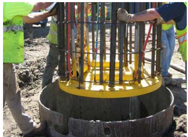
Fig. 5. AFT's tip grouting apparatus being installed in the shaft excavation along with the rebar cage and instrumentation
